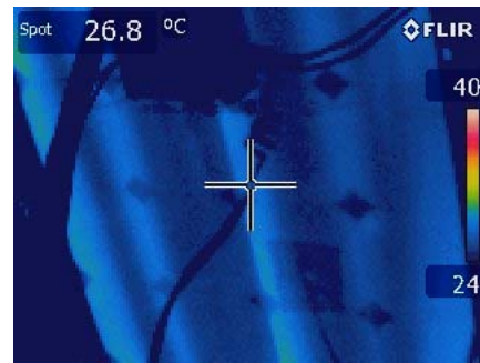
Figure 20. IR image of the PV2 backside
